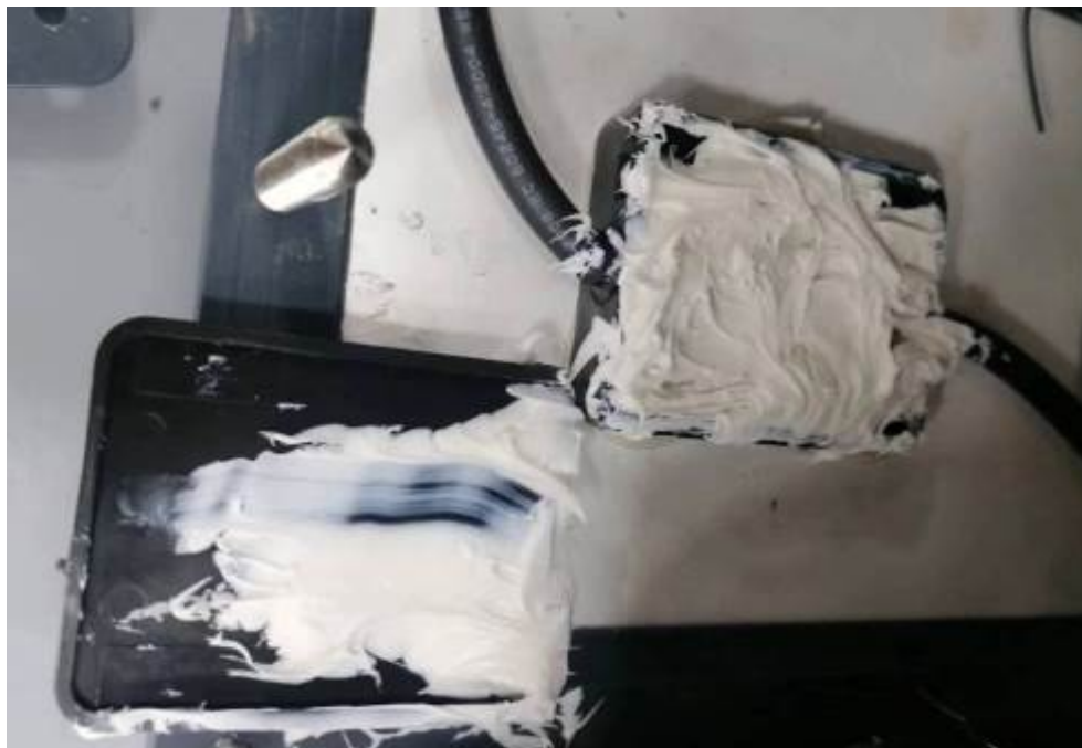
Box internal view of solar panel for W-100
